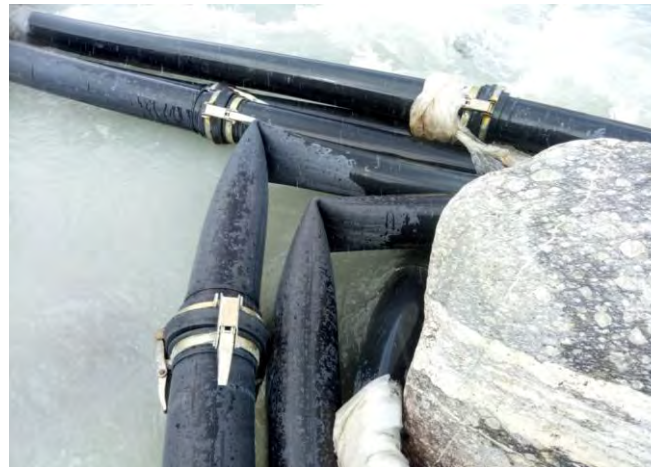
Damage to pipes
