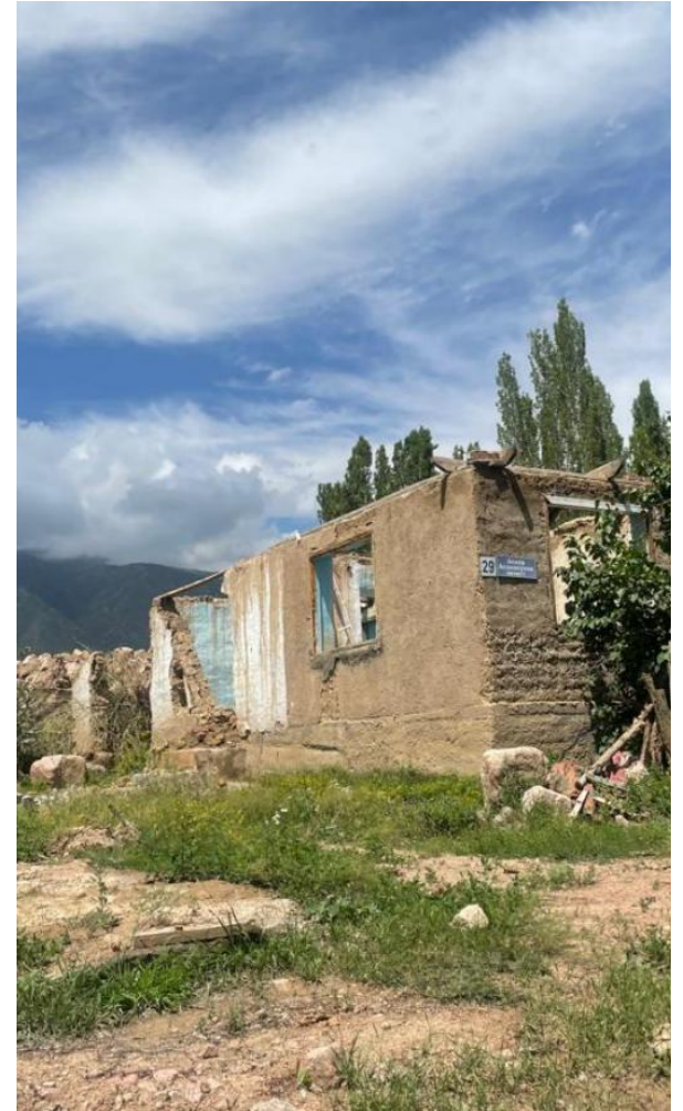
Housing damage following mudslides in Issyk-Kul region, Kyrgyzstan
